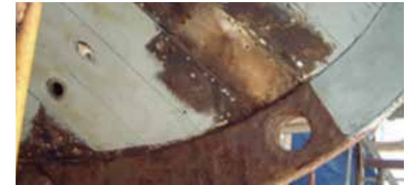
The corroded Hauling plate.
